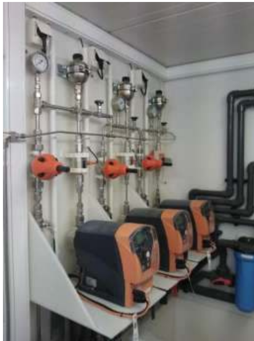
Feeding equipment installed in a container for three different feeding locations in one system
